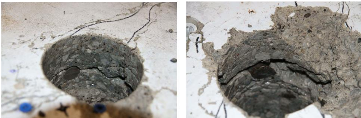
Figure 26. Visible Cover Spalling at Cored Locations
