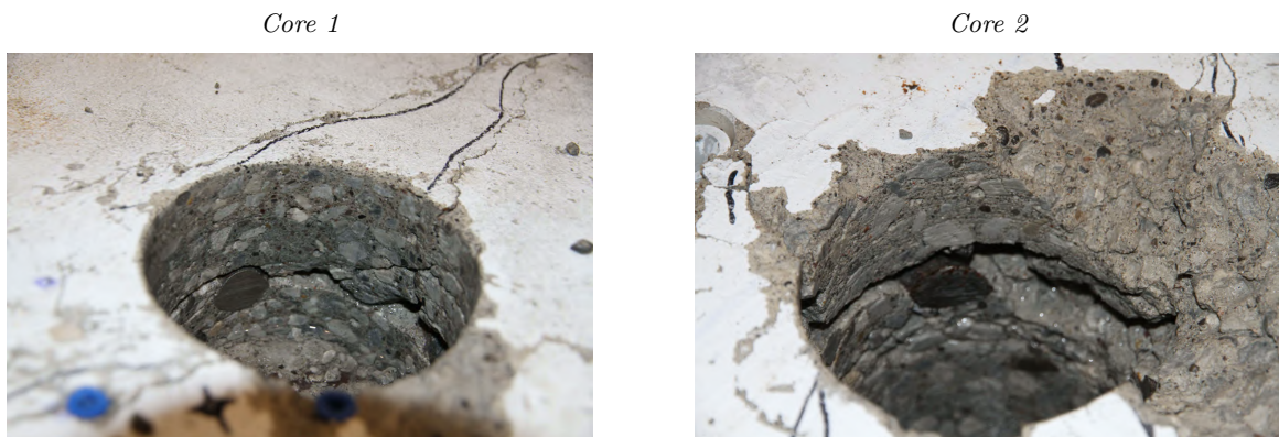
Figure 5.10: Visible Cover Spalling at Cored Locations
