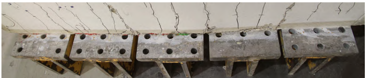
Figure 5.12: Bulging Cover and Residual Curvature in Failed ES1 Specimen (North Face)
