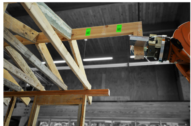
(b) Step 12 in the disassembly sequence. R3 is supporting the remaining roof structure before the start of the reassembly sequence to add additional support.
